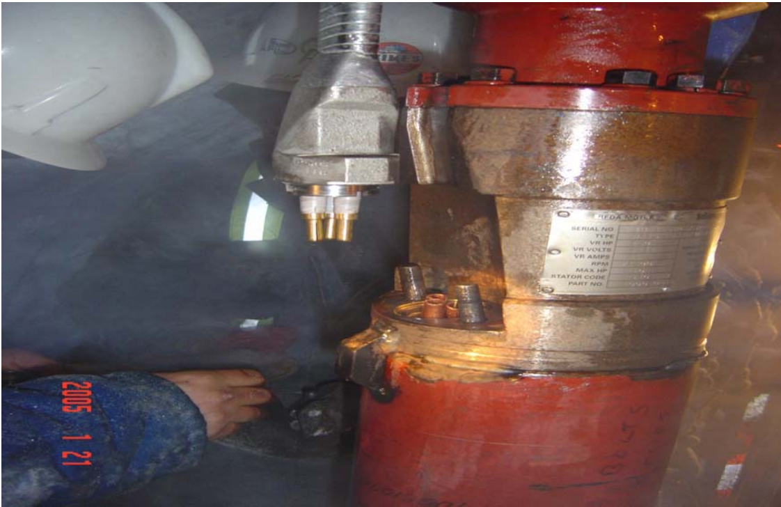
CABLE POTHEAD SPLICE INTO MOTOR HEAD
